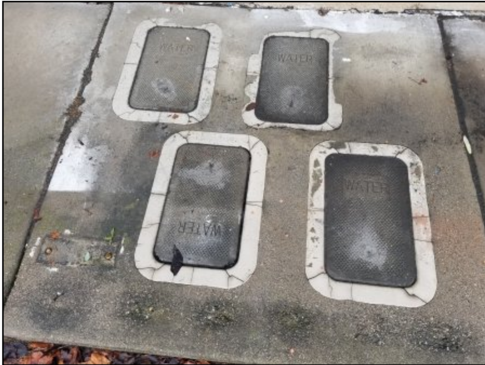
11 : View of the water utilities on the site.
