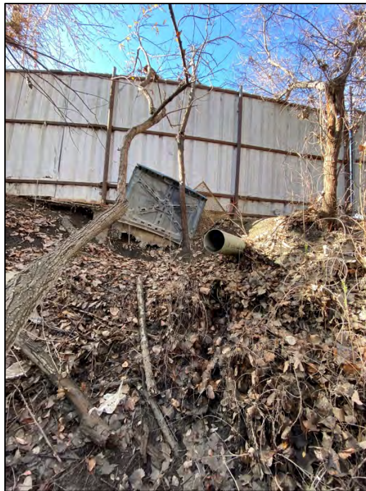
Photograph 6. Drainage pipe that comes from outside the Project Site and drains water into the drainage basin in the northwest corner of the property.
