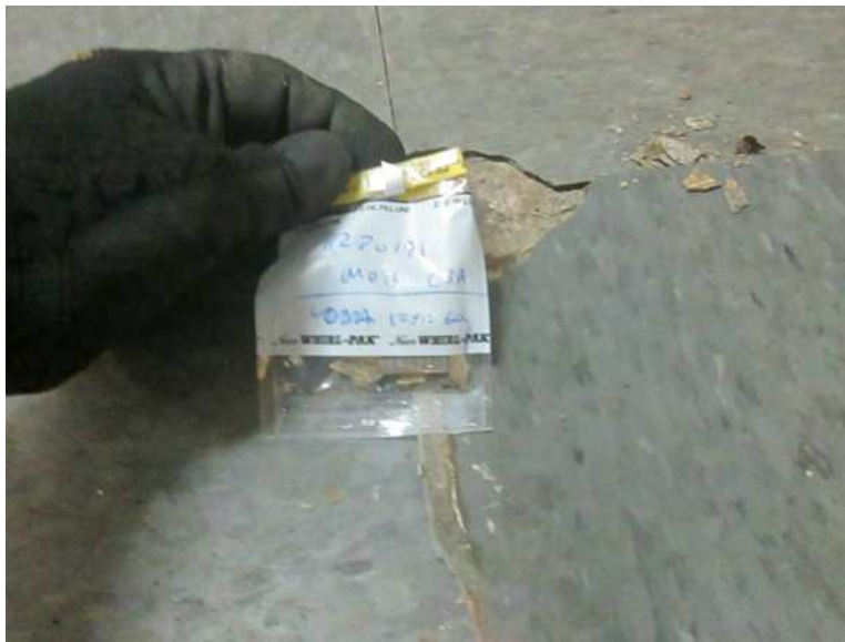
Photo 2 The concrete floors of the building have a gray 12x12-inch vinyl floor tile and mastic that does not contain asbestos.
