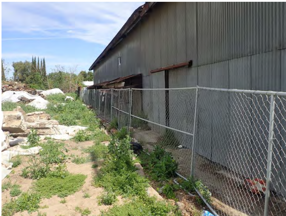
Detail view of west elevation at demolished San Jose Foundry site, viewed facing north.
