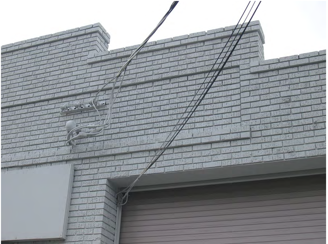
Detail view of brick detailing on façade at 151 North Autumn St., viewed facing southwest.
