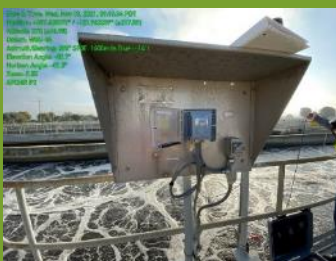
New transmitter installed at the Nitrification Tank Gallery A.
