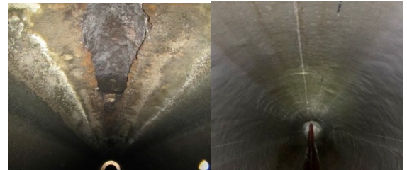
96-inch primary effluent pipe with crown corrosion before (left) and after (right) CIPP rehabilitation.
