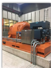
Tertiary Building blower after a motor replacement.
