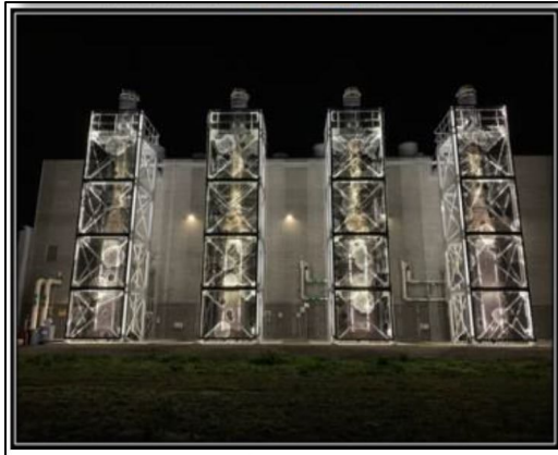
FIGURE 14 THE NEW COGENERATION BUILDING AT NIGHT, BEGAN OPERATION IN 2021
