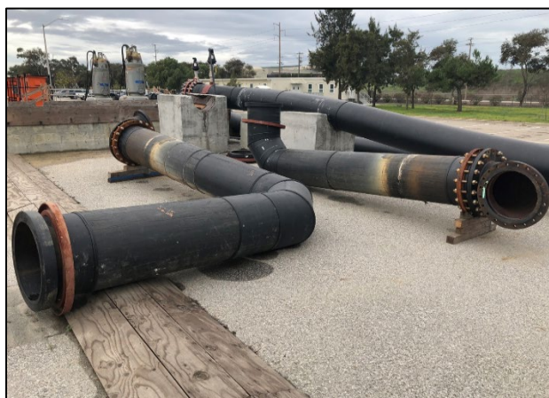
FIGURE 21 SECTIONS OF 36-INCH HDPE PIPE, USED AS A TEMPORARY PIPING SYSTEM IN 2018 THAT WILL BE USED AGAIN FOR THE SES REHABILITATION PROJECT
