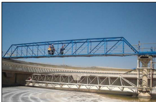
FIGURE 28 WORKER ON A CLARIFIER "TOW-BRO" ARM
