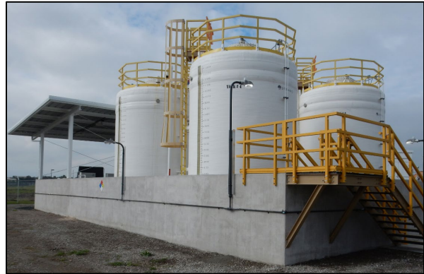
FIGURE 17 IRON SALT FEED STATION
