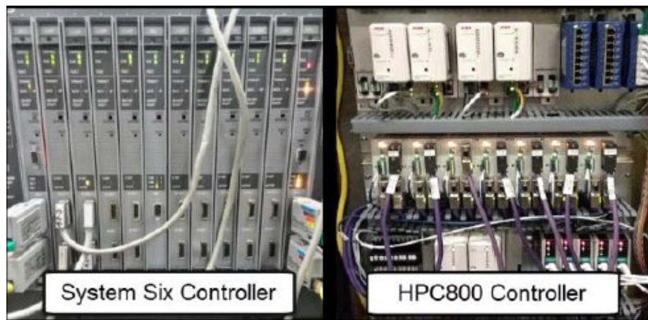
FIGURE 31 THE DCS IS BEING UPGRADED FROM SYSTEM SIX (LEFT) TO NEW HARMONY (RIGHT) CONTROLLERS
