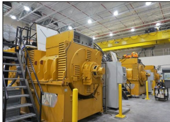
FIGURE 15 NEW COGENERATION ENGINES INSTALLED IN THE NEW COGENERATION BUILDING
