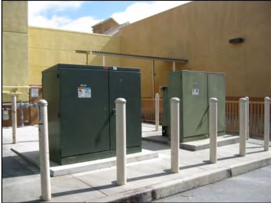
Pad-mounted transformers on south side of building.
