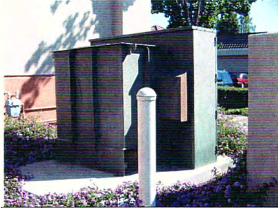
Photo #14: Typical pad-mounted transformer
