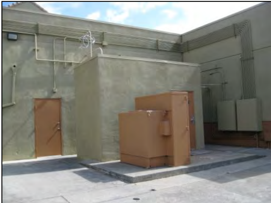
Pad-mounted transformer on south side of building.
