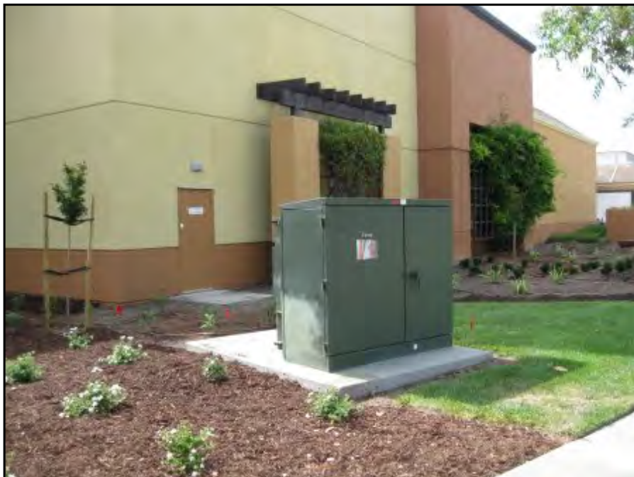
Pad-mounted transformer on west side of Dick's Sporting Goods.
