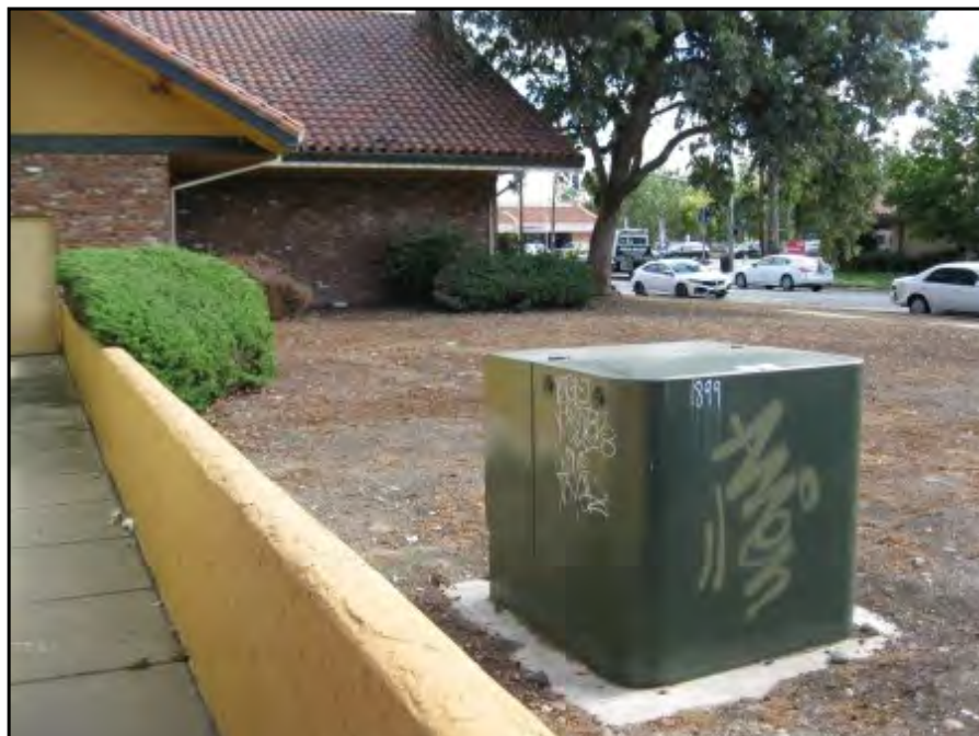
Pad-mounted transformer on southeast corner of Marie Callender's (620)
