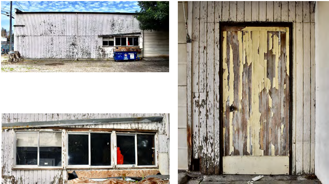
Figure 15: south side shop wing (upper right), windows close-up (lower left), pedestrian door (right)
