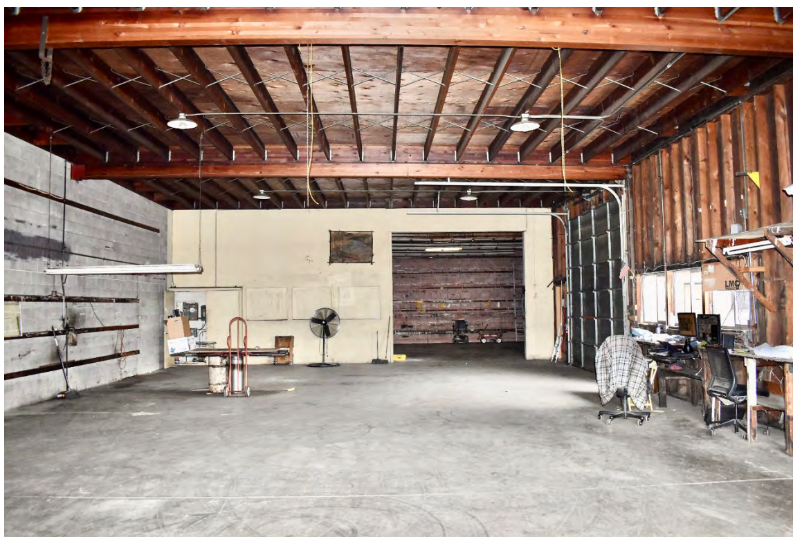
Figure 13: Shop wing, view toward the rear. Note the three covered windows to the left of the opening to the warehouse/office wing
