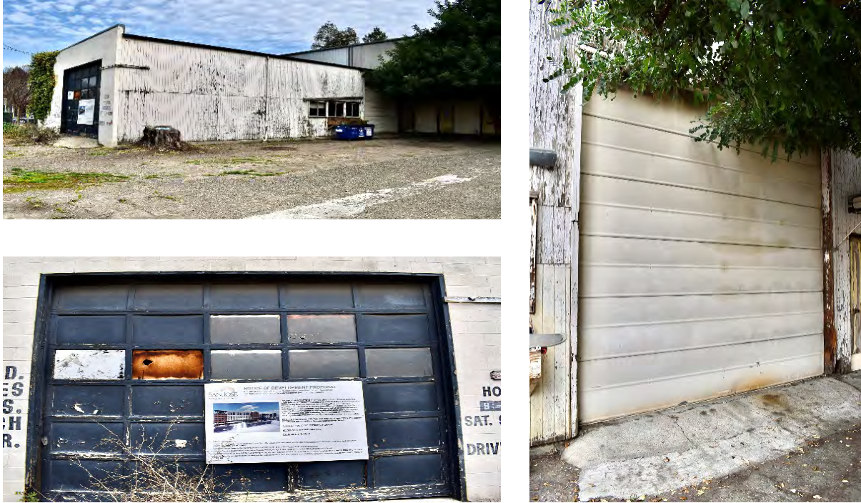
Figure 14: location of both rolling doors (upper left), wooden door (lower left), metal door (right)
