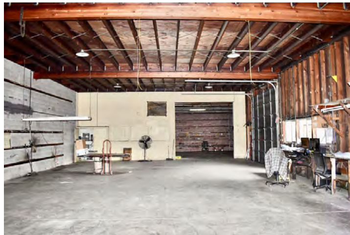
Shop wing, view toward the rear. Note the three covered windows left of the opening.
