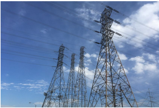
Electrical grid transmission towers in Pasadena, Calif., Aug. 15, 2020.
