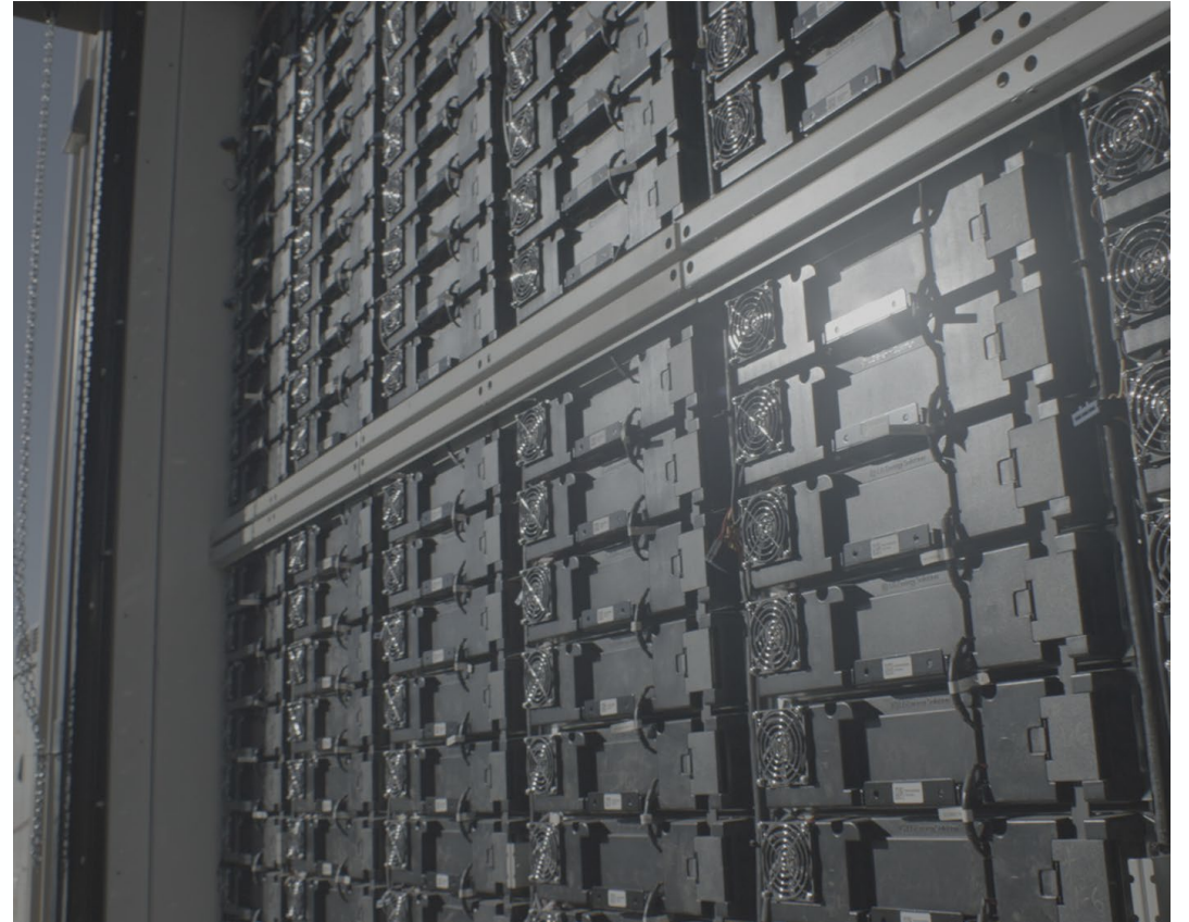
Battery storage from SJCE's Kern County Solar and Storage Project
