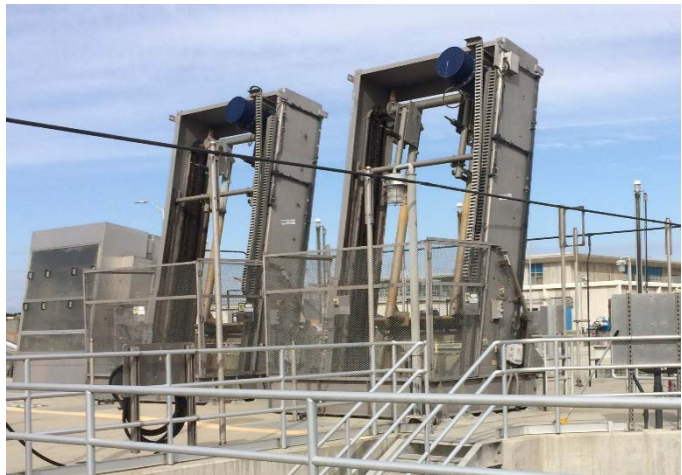
Headworks 1 Bar Screens
