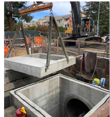
Top of Precast PCC vault
