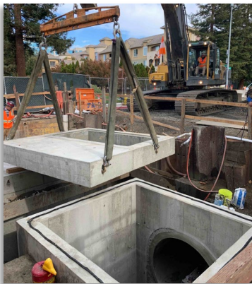
Top of Precast PCC vault
