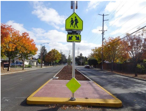
Safety Improvements along McLaughlin Avenue consisting of raised median islands, ADA ramps, and flashing beacons
