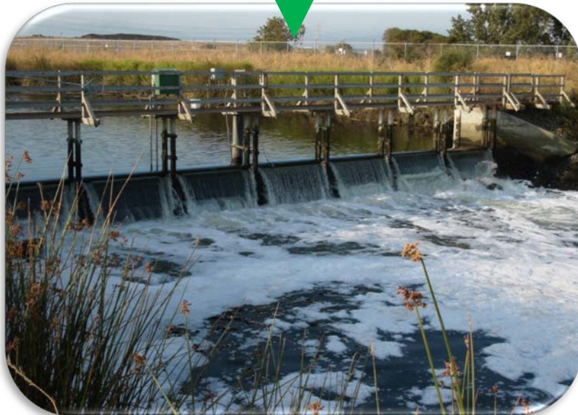
Treated water flows to the Bay!
