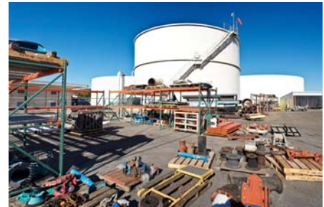
Digester Tanks at the Water Pollution Control Plant Photo by Robert Dawson
