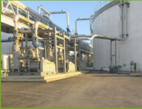
Gas compressors, left, will help mix gas in the digesters.
