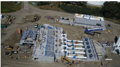
Aerial view of the new Raw Sewage Pump Station and Grit Facility.
