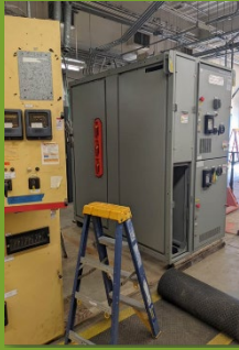
One of two newly installed spare breakers for the S40 switchgear.
