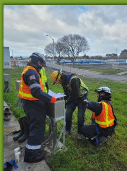
Measurements being taken at Secondary Battery A.
