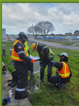
Measurements being taken at Secondary Battery A.
