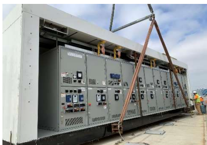
New M4 Switchgear Installation
