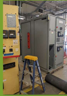
One of two newly installed spare breakers for the S40 switchgear.
