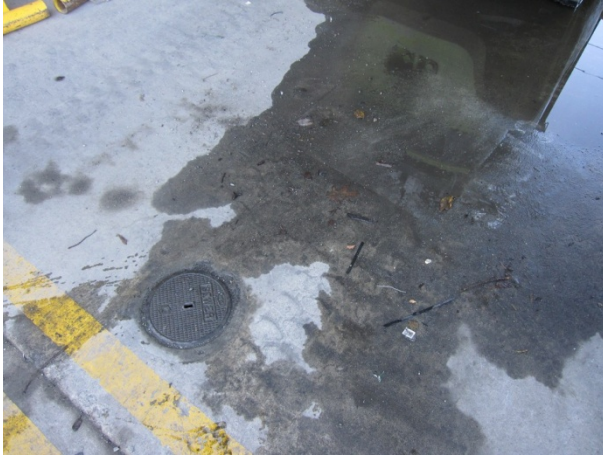
Photograph 7. Concrete-filled oil-water separator at AT&T (below standing rain water).
