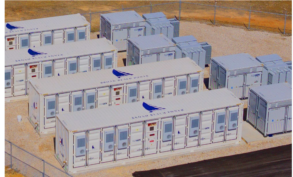
Source: Broad Reach Power website
