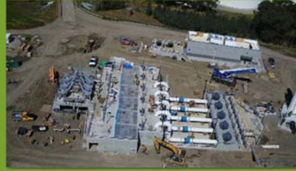
Aerial view of the new Raw Sewage Pump Station and Grit Facility.
