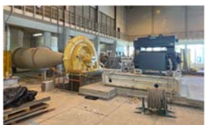
New motor installed on Secondary Blower #2
