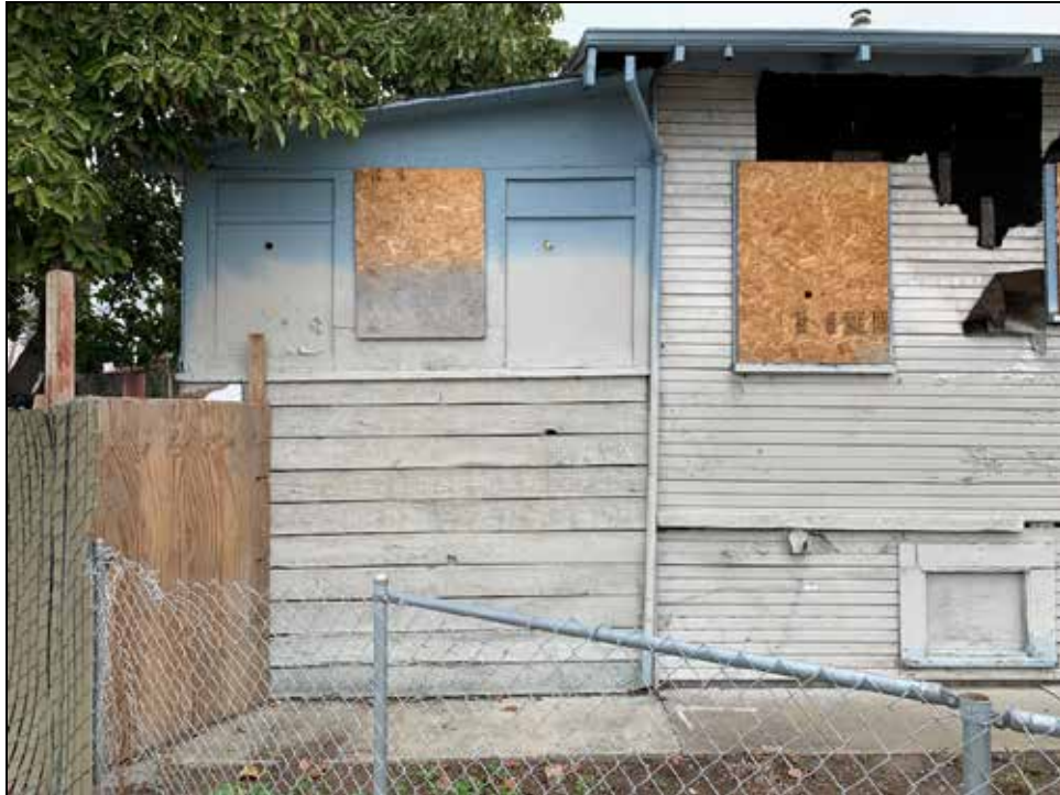
Photograph 6: Rear north end of west elevation, showing rear addition; facing east, January 18, 2022.
