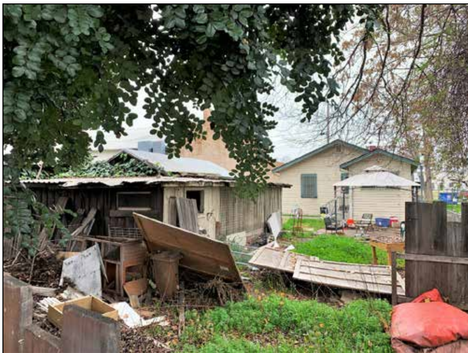
Photograph 3: Rear north side of residence and northwest corner of detached garage and shed; facing southeast, January 18, 2020.
