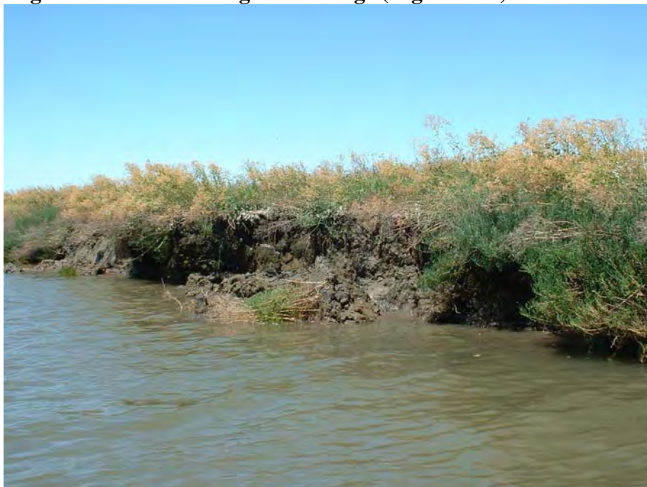
Figure F-4. Scour Along Marsh Edge (Segment 15).
