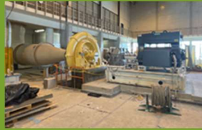
New motor installed on Secondary Blower #2.
