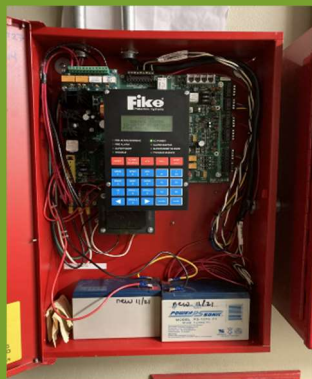
Typical Fire Alarm Control Panel
