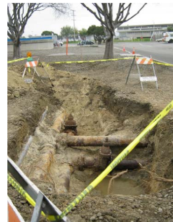
Underground pipes are common at the Plant.
