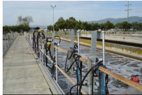
Aeration Study sensor equipment (handrail rack with rotameters)
