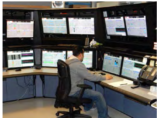
Phase I: Operator Juan Zepeda using improved graphic displays in the Control Room.
