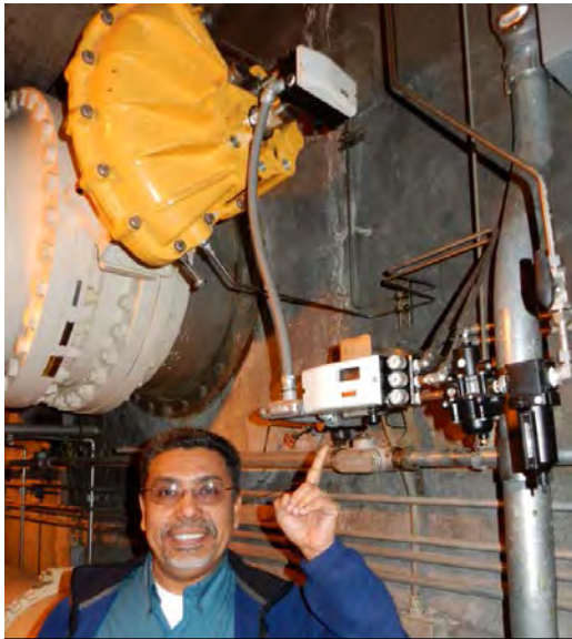
Senior Process Control Specialist, Carlos Garcia, points to an ABB Valve Regulator collecting signals from a 36" influent valve.
