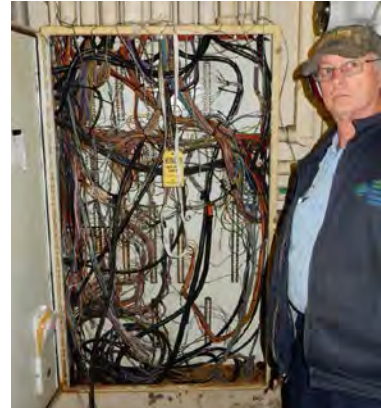
Where to start? Instrument Tech, Don Samuel, with a 20+ year-old electrical cabinet.
