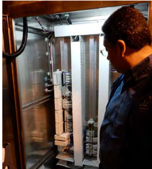
Cleaner cabinet: Signals from the Valve Regulator are wired as I/O points to I/O cards.
