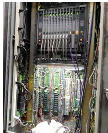
DCU Cabinet #7: DCI System Six on top; old original wiring at bottom. All will be replaced in Phase III.
