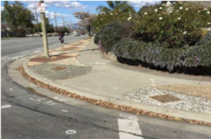
Missing – No ramp present
