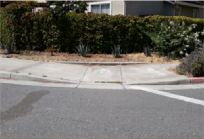
Substandard (Low Barrier) – Accessible but missing detectable warnings
