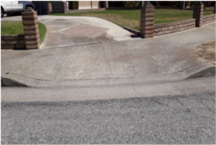
High Barrier – Side flares and running slope out of specification
