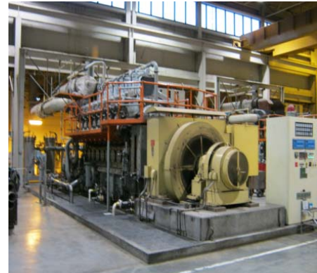
Existing Engine Generator, EG-2
