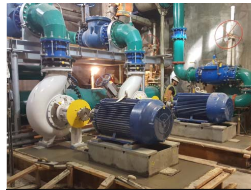
New Sulzer pumps.
