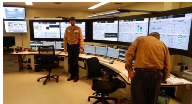
Ops. Forepersons, Candelario Sepulveda and Brian Boardman at work in the new ABB Computer Room.
