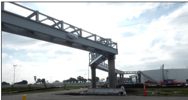
New permanent above-ground piping racks: “The Monorail.”
