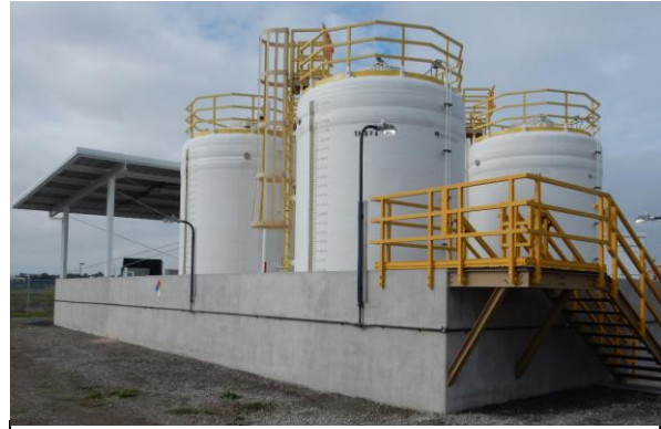
Iron Salt Feed Station.
