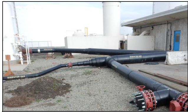
Temporary digester gas above-ground piping
