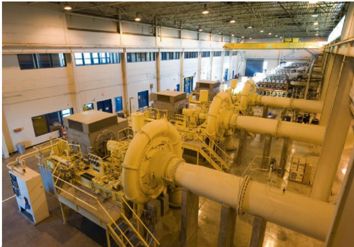
Process Air Blowers, PAB-1 thru PAB-3.
