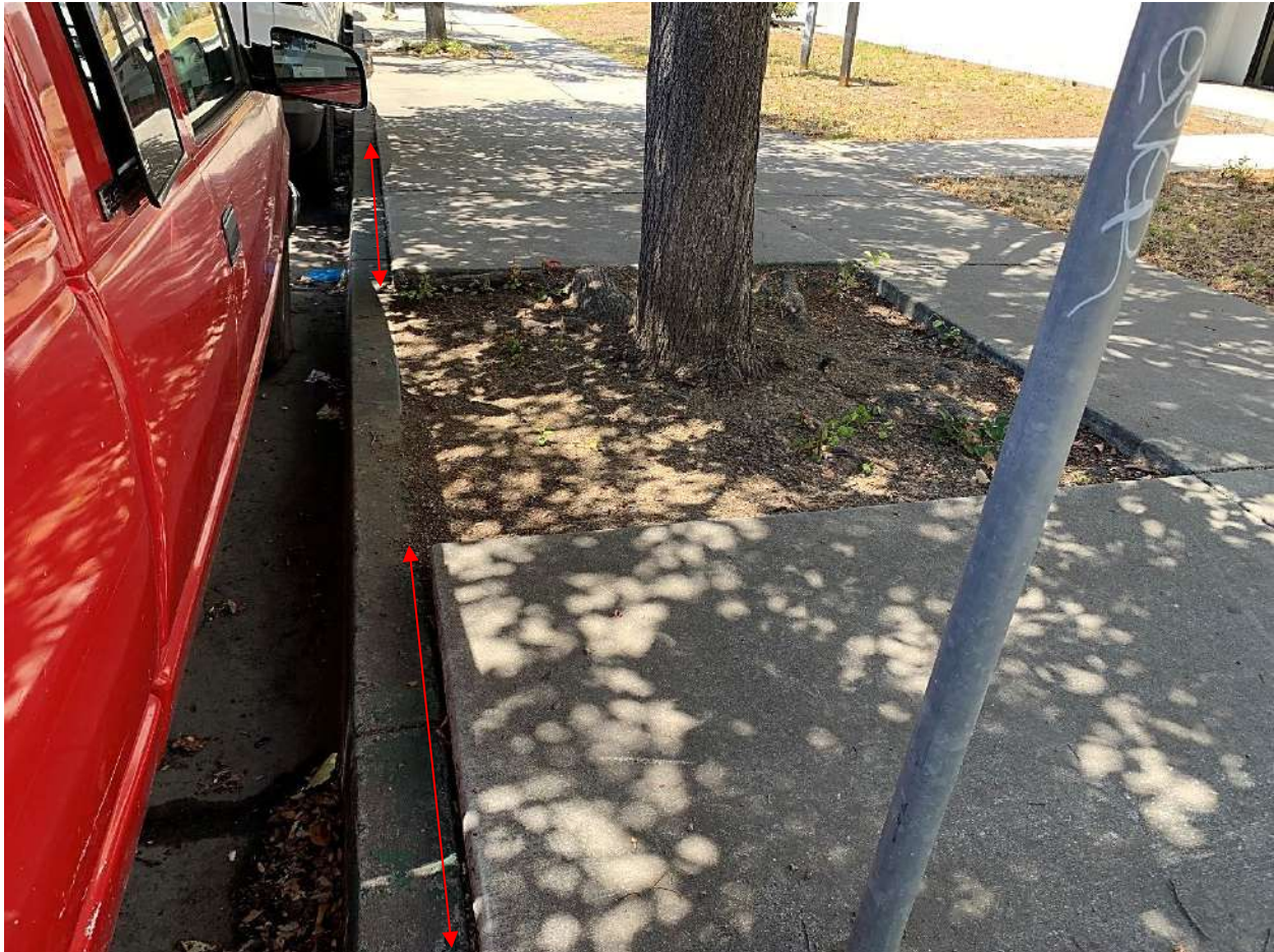
Image #7 – Tree T17, ornamental pear. Note sidewalk lifting.
