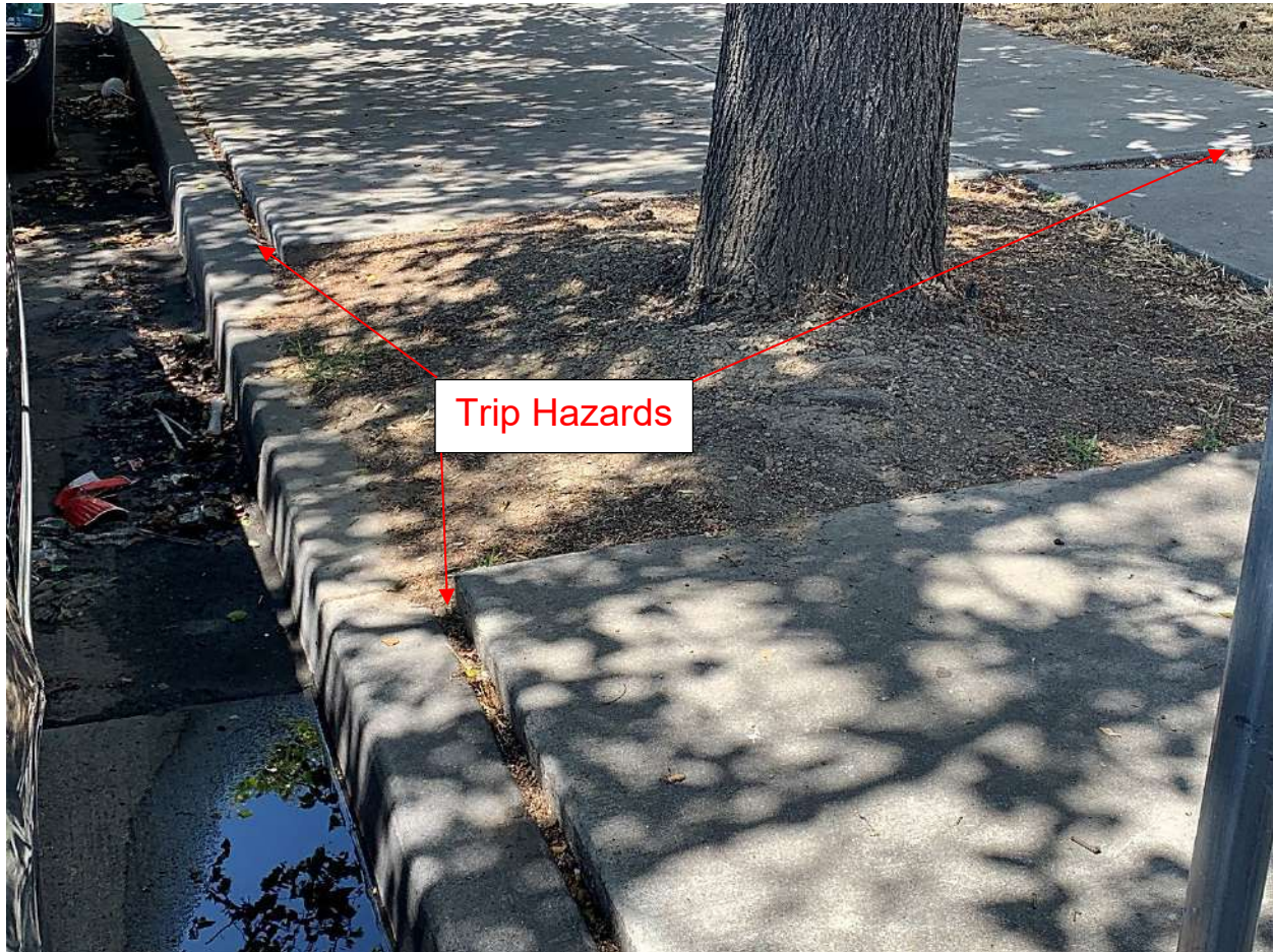
Image #6 – Tree T16, ornamental pear. The lifted sidewalk is creating significant trip hazards in three locations.
