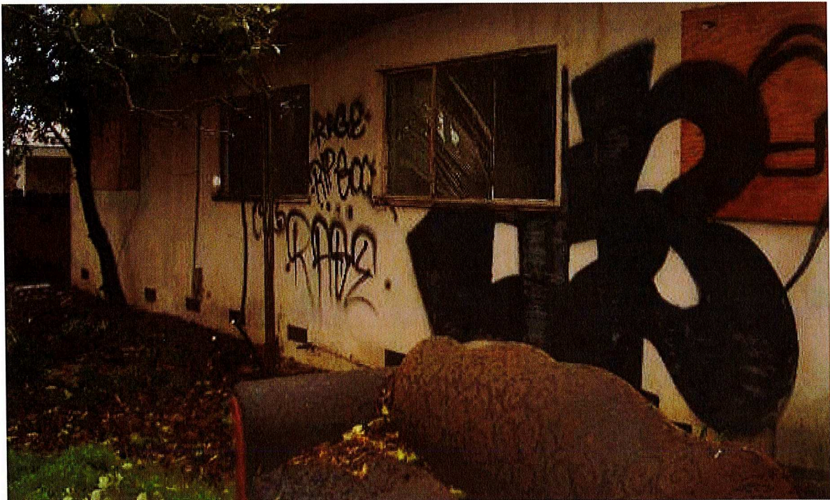
1-28-21 Two rear windows to home unsecured
