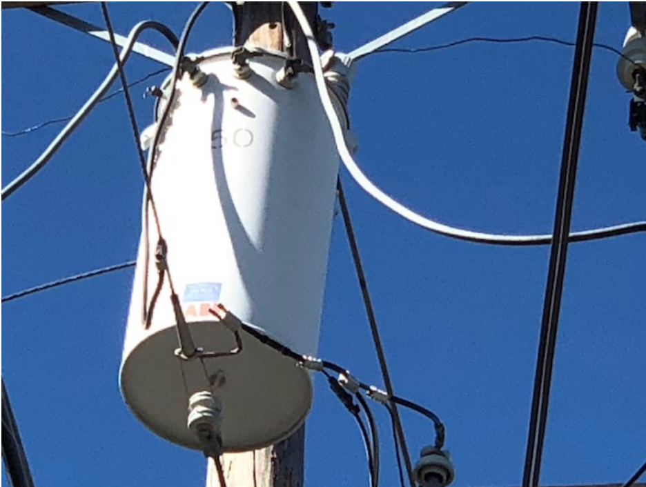
Photograph 13. Pole-mounted transformer labeled non-PCB.
