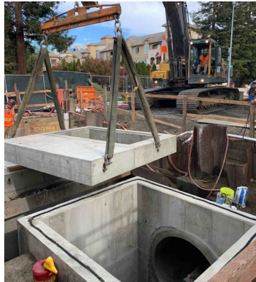
Top of Precast PCC vault
