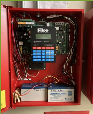
Typical Fire Alarm Control Panel
