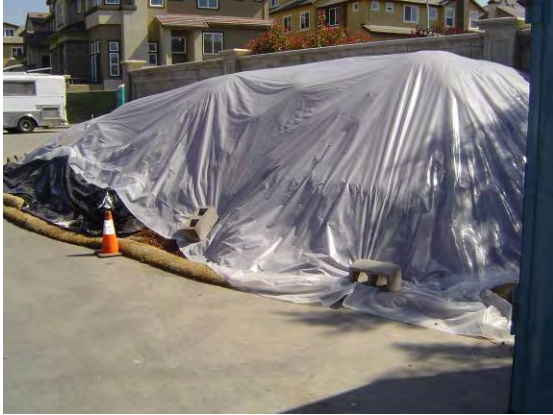
Construction materials covered and contained to prevent runoff pollution on Lundy Avenue.
