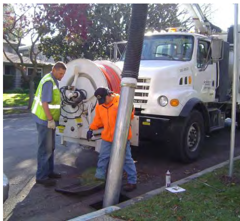
Department of Transportation crew cleaning a storm drain catch basin in a neighborhood near Almaden Lake Park
