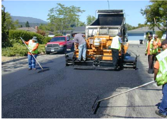
Department of Transportation paving crew applying their training along with the pavement
