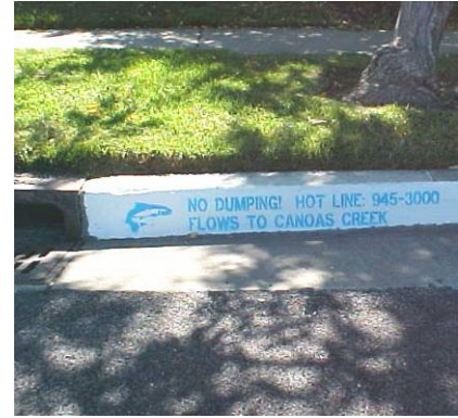
Storm drain inlet stenciled with hotline number and local creek name.
