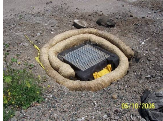
Proper storm drain protection during construction prevents construction debris and sediment from entering the storm drain.
