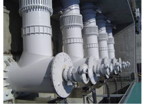
Pumps at the Rincon II Pump Station.
