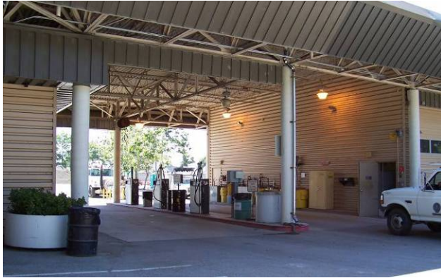
Fuelling island at Mabury Corporation Yard.
